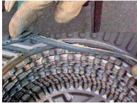
When old glue and gaskets are not completely removed, insufficient sealing is the result. This creates a high risk of leakage.
